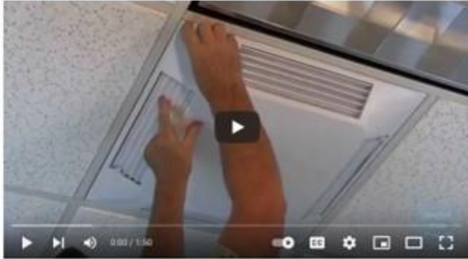
Comfort First Introduction and Installation
